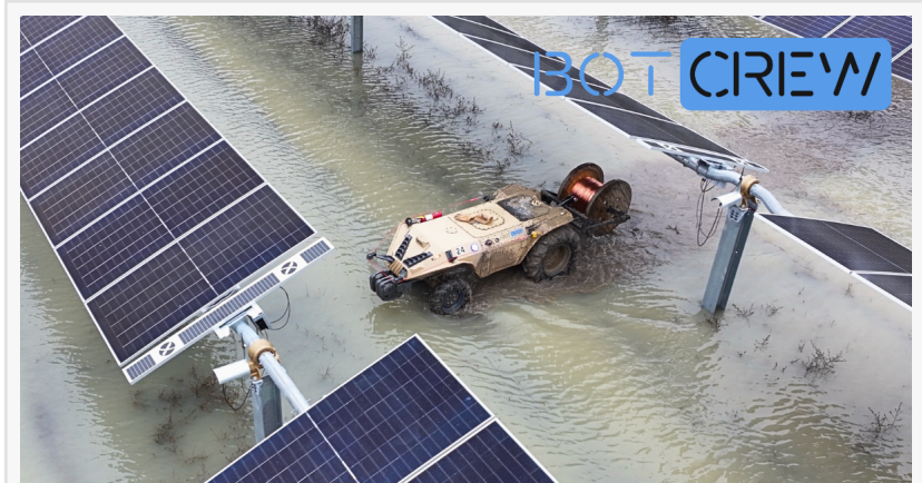
BotCrew's Gravion robotic platform operating on a utility-scale solar construction site, designed to support day-to-day workflows in challenging field conditions.
