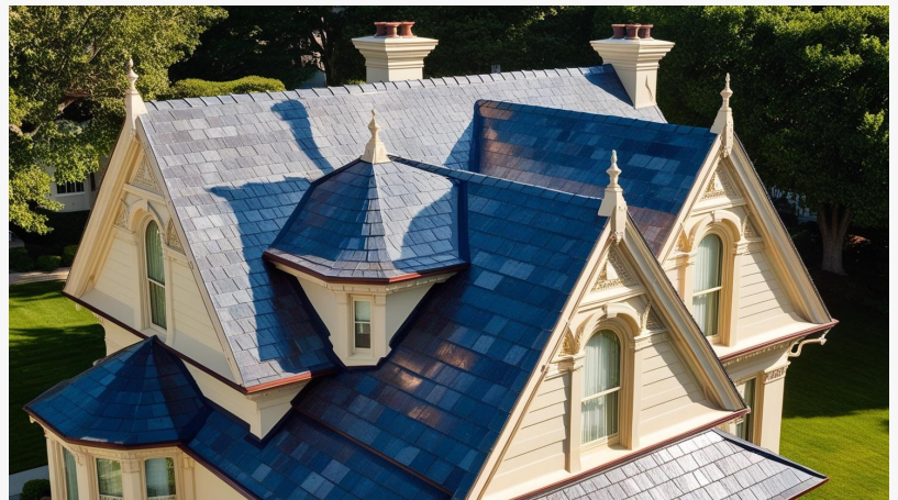
Storm Damage Assessment
