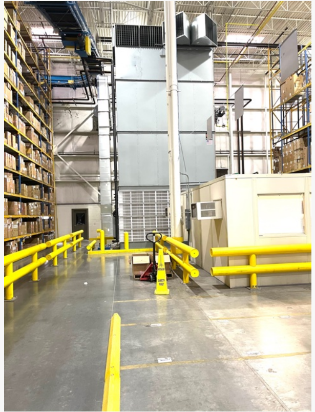
PVH Distribution Center Environmental Control Unit
